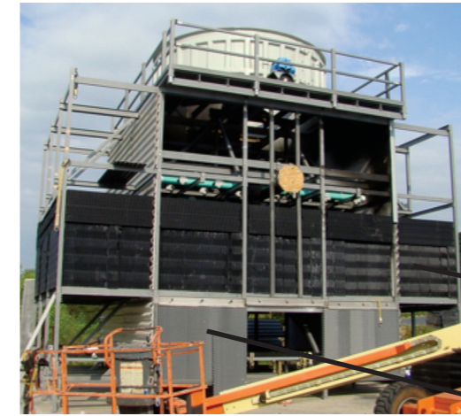
Series ES test cell under construction with standard PVC fill, eliminators, and WST inlet louver panels
