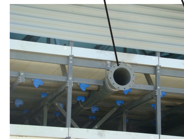
Fire-retardant water distribution system header.
